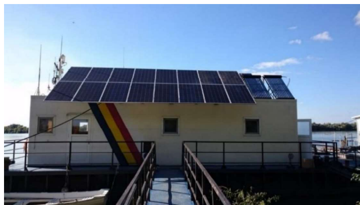
Fig. 3 Surveillance pontoon endowed with solar energy solutions
