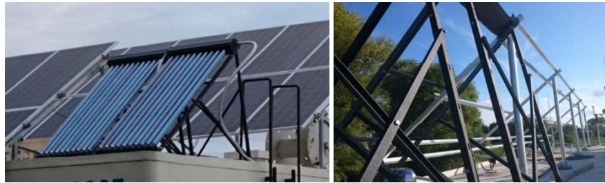
Fig. 4 Solar panels and mounting rails on the roof of the pontoon
